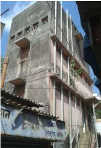
The lack of space in slums often leads to two and three stories to produce the number of seats the settlement requires even when the ratio of seat to persons is 1 seat for 50 people.
