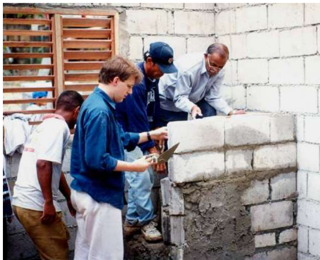
Jockin helping in the construction of the model house for the Security of Tenure launch in Payatas, the Philippines, 2000
